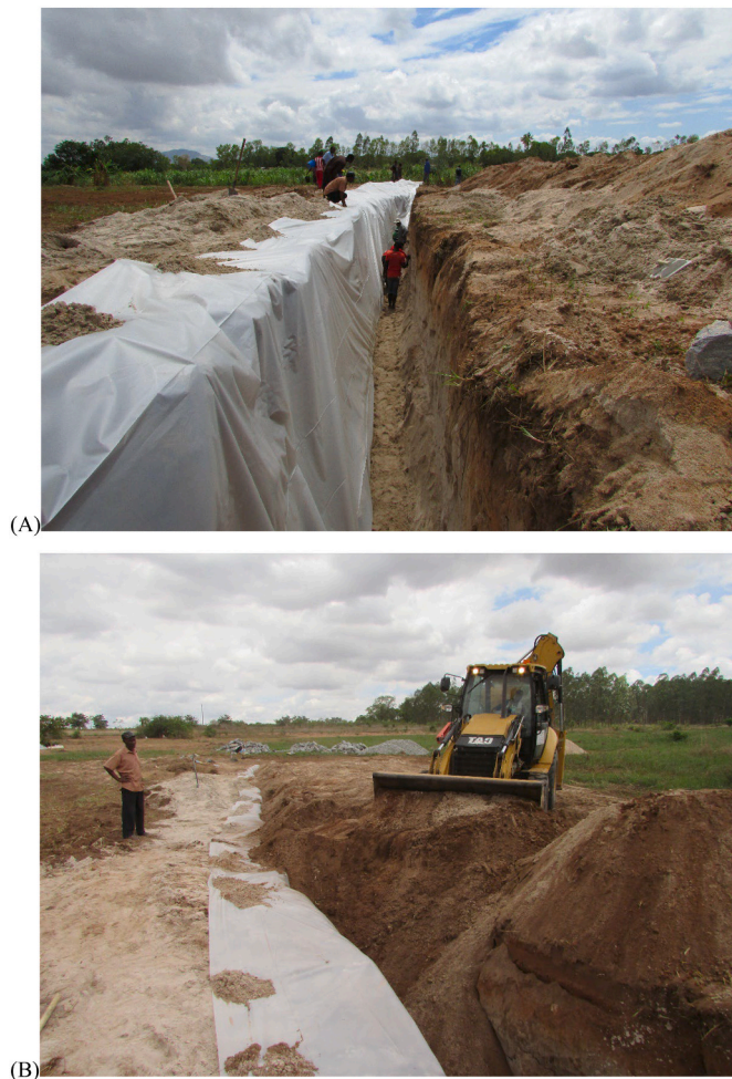
Fig. 1. Underground dam construction process, showing: (A) The trench dug across the drainage line, with the outlying wall covered with plastic sheet; and (B) A tractor filling the trench with the earth that was previously removed. Source: Flávio A. Marques.
